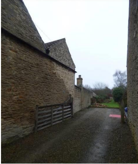
Further general view of west elevation to applicant's property. Note also applicants guttering which overhangs neighbour's property.
